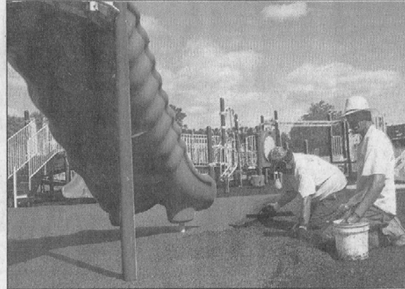
FUN ON THE WAY: Tomas Hernandez, foreground, and Jose Alvidrez spread surface coating on the Fun For All Playground Saturday at the Warrenton Aquatic & Recreation Facility in Warrenton.
